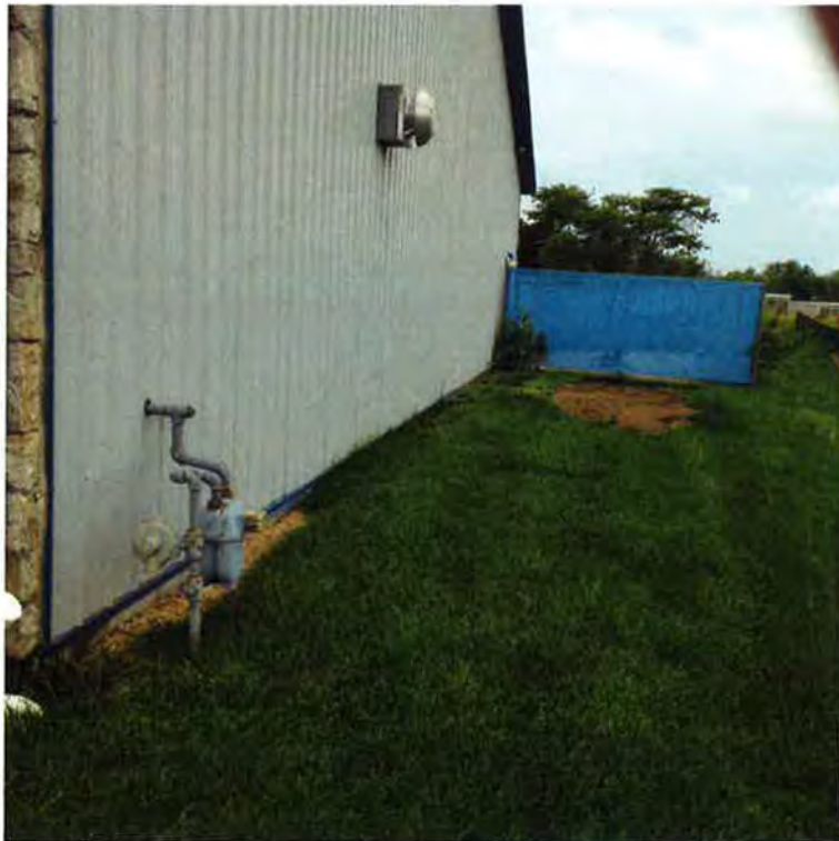
Photo 2. Facing south along Rudroff Building – no utilities along existing easement to be vacated
