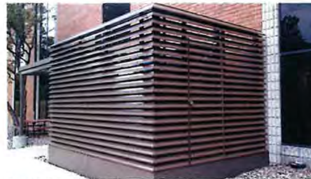
FIGURE 1.12 EQUIPMENT AND TRASH SCREENING EXAMPLES
